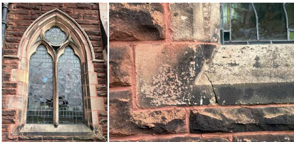
Nave south elevation window – cracked cill
