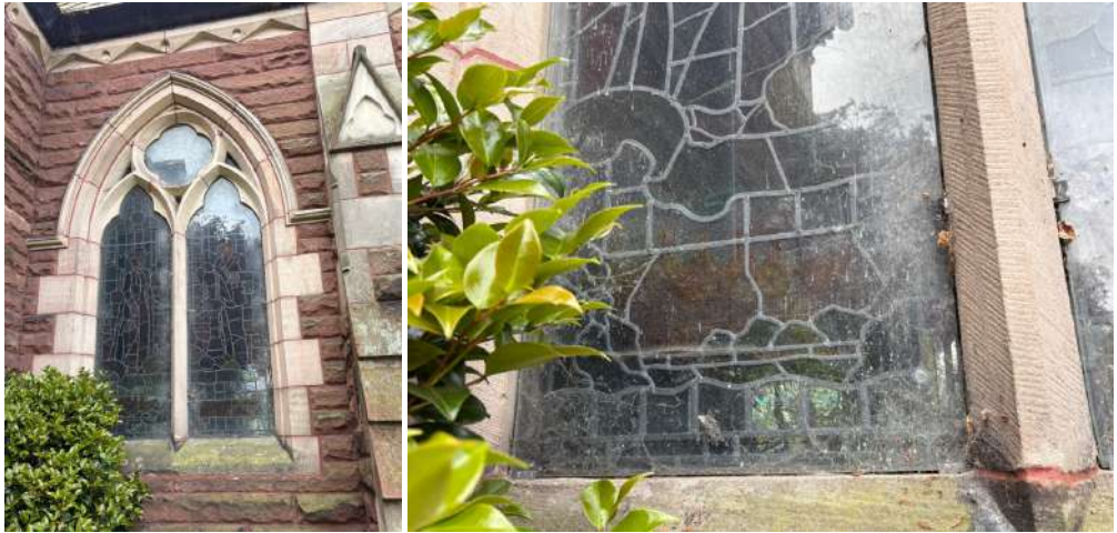
North nave windows and dirt / debris behind polycarbonate
