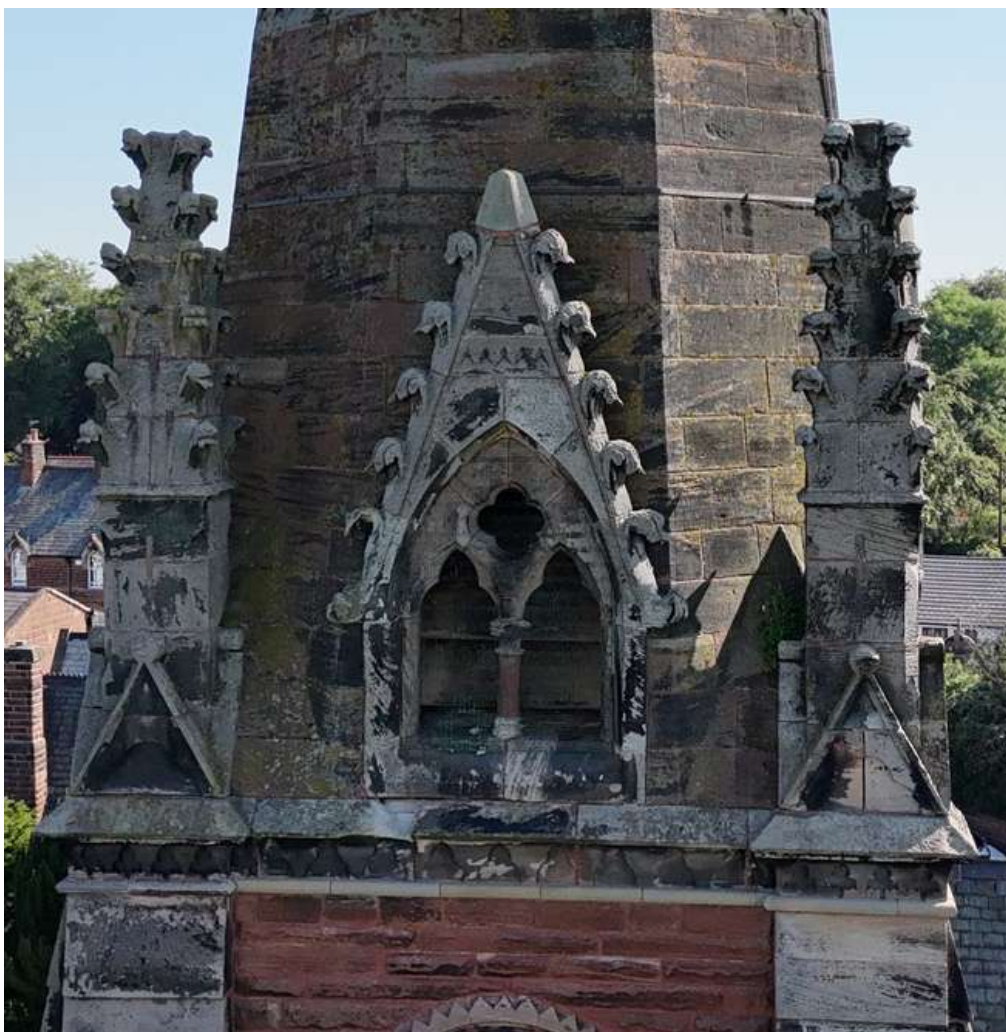
South side – at the base of the louvred opening can be seen the damaged stone, from which a loose section was removed during the recent steeplejack inspection.
