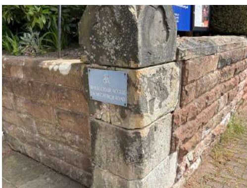
Damage to southern gateposts
