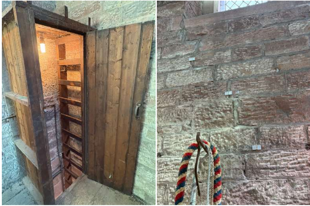
Sounding chamber – access point and old crack on wall
